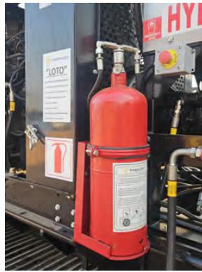
FIRE SUPPRESSION SYSTEM
