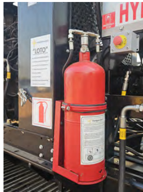
FIRE SUPPRESSION SYSTEM
