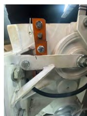
WIRELINE WINCH LIMITER
