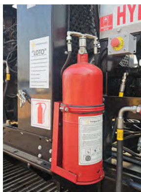
FIRE SUPPRESSION SYSTEM
